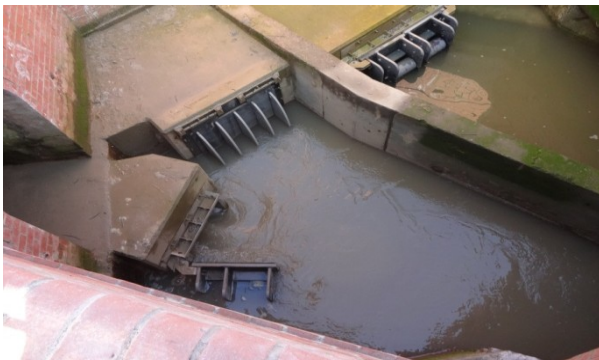
Figure 5 Leiston drain sluice gates working
