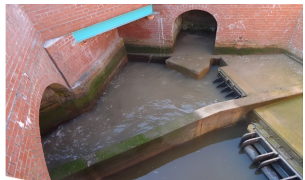
Figure 6 New Cut sluice gates
