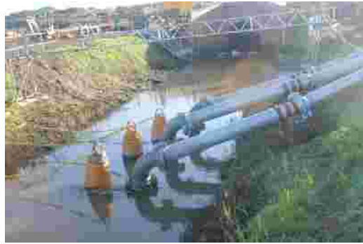
Three pumps in New Cut for discharge to sea.
